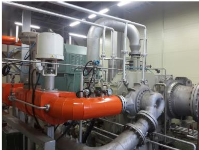
TurboTech Turbine at Waste Incineration Plant in Korea
